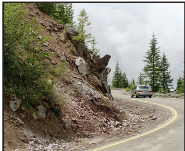
Figure 15 — Loose rock rubble from top of the 40,000-year-old Ricksecker Point lava flow. USGS photo by C. Driedger.
